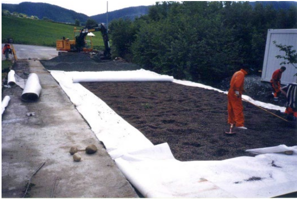
Figure 1.1.13. Frost insulation using expanded clay lightweight aggregate at Sandmoen test field in Trondheim (copyright ROUGH project participants).
