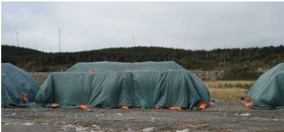
Figure 3.2.2: Tarpaulin installed on top of a pile of GBR-C for site storage (photo courtesy Terrafix Geosynthetics)
