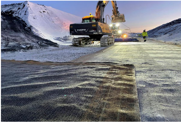
Figure 1.1.3. Geosynthetic Clay Liner under cold climate installation, mining application Finland Jan 2022 (copyright ROUGH project participants).
