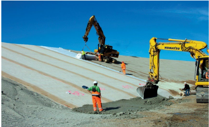
Figure 1.1.16. Filter in a rip-rap erosion protection in water reservoir (copyright ROUGH project participants).
