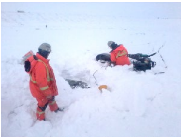
Figure 3.3.1: Example of GBR covered by a 500 mm snowfall before completing installation (Courtesy FC Geosynthetics)
