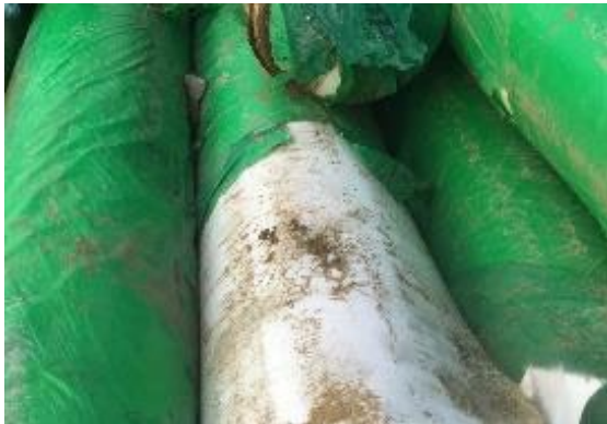
Figure 2.2.1. Examples of tear of the wrapping which may lead to water entering in the roll and then freezing.
