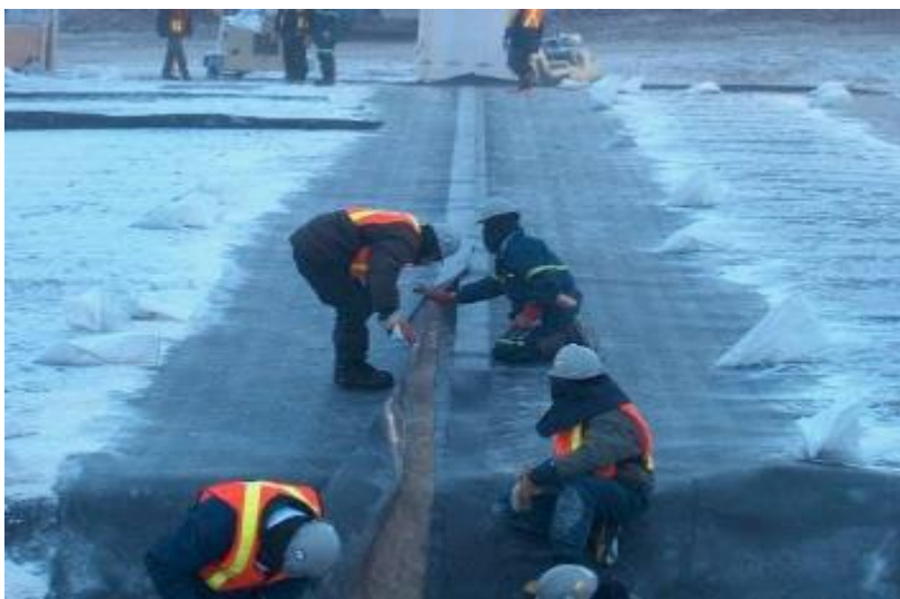
Figure 3.2.5: Controlling cleanliness of both sides of the geomembrane being welded together (photo courtesy of A&A Technical Services)
