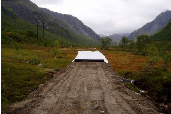
Figure 1.1.5. Construction of access road on peat subsoil in Lofoten, Northern Norway (copyright ROUGH project participants).
