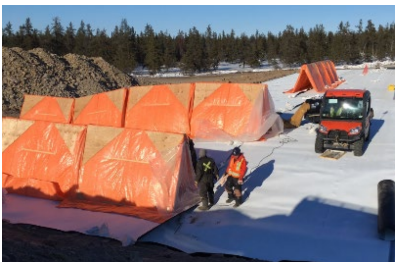
Figure 3.2.6: Use of tents to control environmental conditions and reduce humidity around a seam (photo courtesy of A&A Technical Services)
